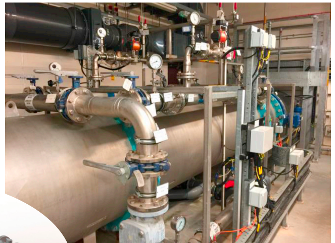
GDS installed at customer site
